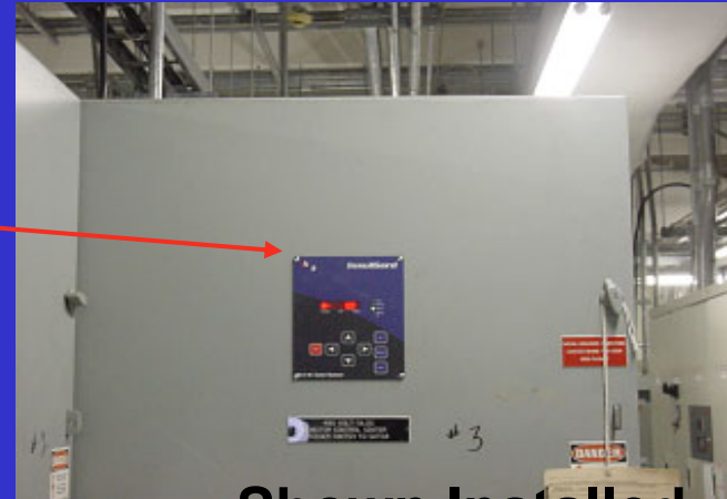
Shown Installed on front door
