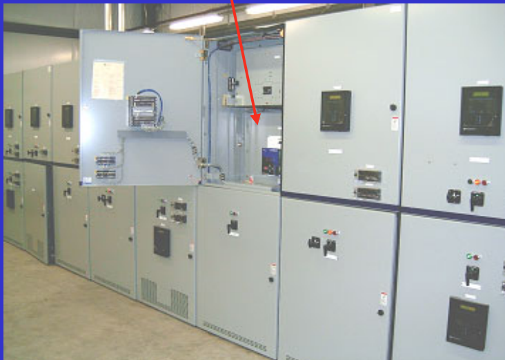
Shown Installed inside the compartment
