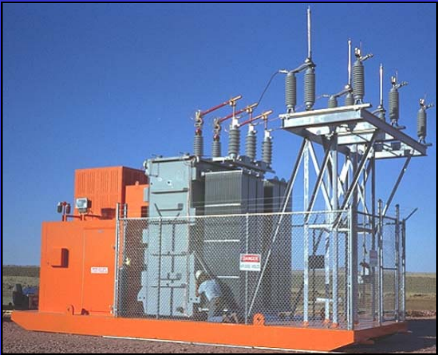
Skid Mounted Substation
