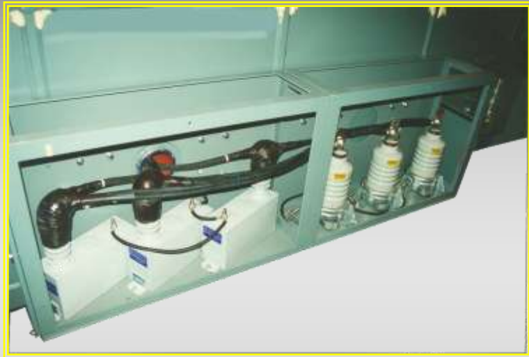
HV Junction Box With Surge Caps & Arrestors
